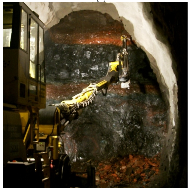
Figure 3-2: Mixed face from Fáskrúðsfjörður tunnel. At the top there is sediment underlain by a thin basalt layer, then another sediment layer and finally scoria from the middle to the bottom [46].
